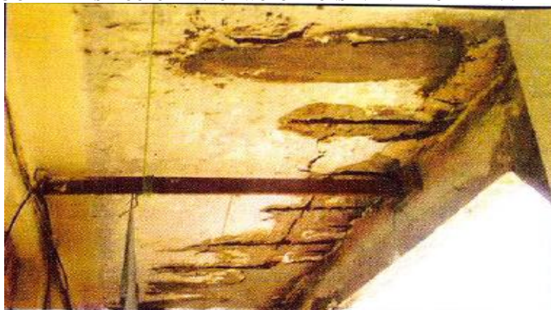
FIGURE 2 CORROSION OF STEEL AND SPALLING OF CONCRETE IN A RCC CANOPY
