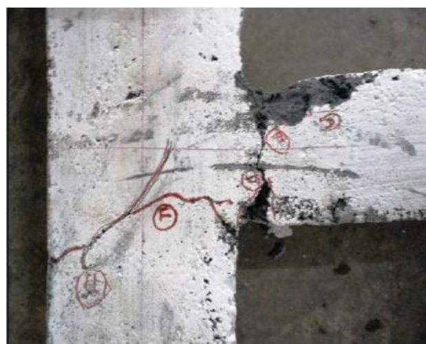
(b) CRACK PATTERN ON FACE B
